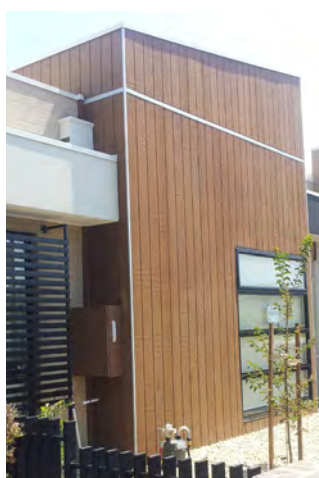
The board shows signs of lightening.
